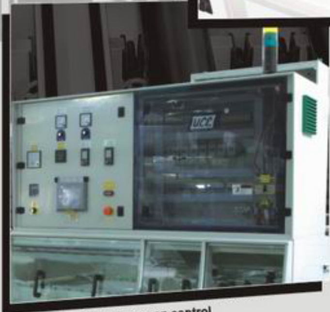
PLC and touch screen control
