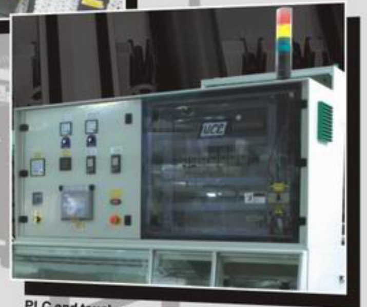
PLC and touch screen control
